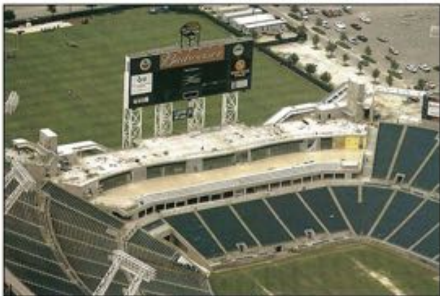
This July 2003 photo shows construction of the $46 million renovation to ALLTEL Stadium. New to the south end zone are the Bud Zone sports bar, a 700-seat Terrace Suite, an open-air Patio.
